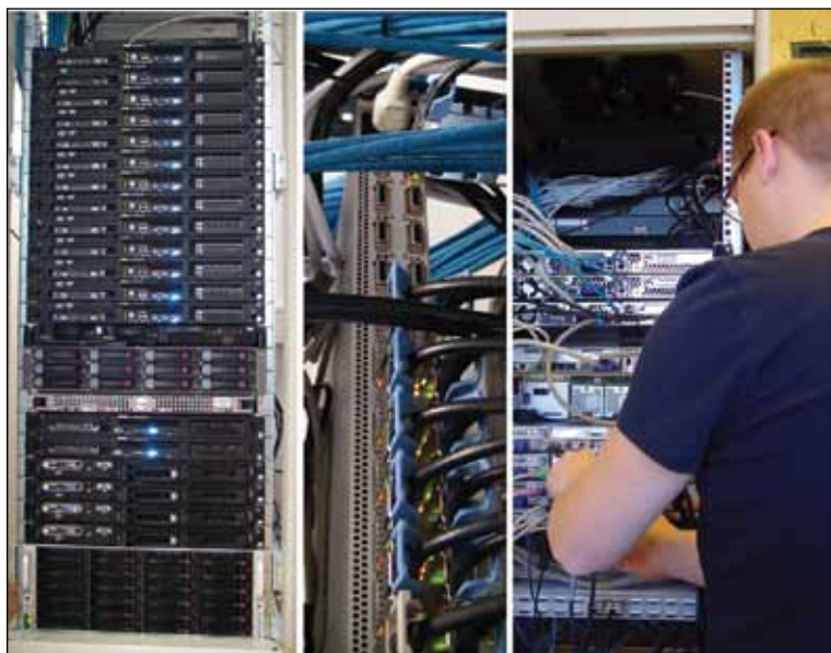
Cloud computing physical infrastructure: servers, storage, Infiniband switch
